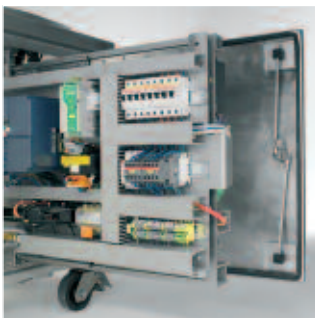
Control hardware arranged for easy maintenance.
